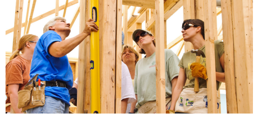
Trained staff supervise home construction, with volunteers and partner families contributing most of the labor. (Photo: James Nedresky)
